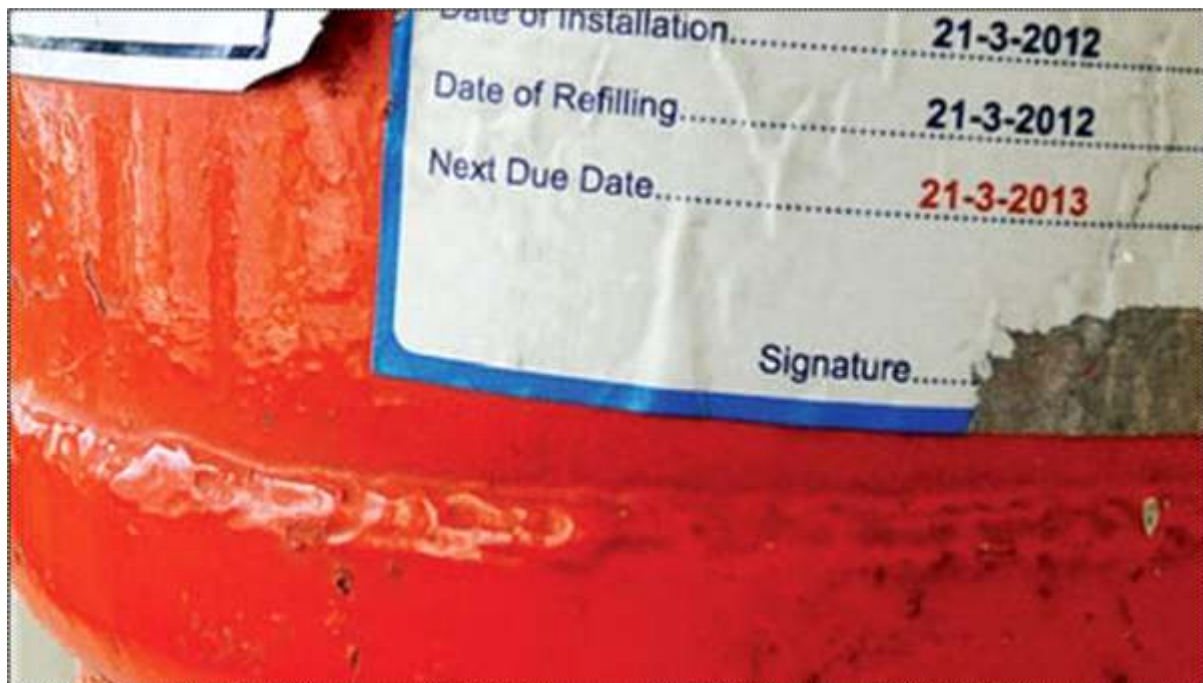
Fig 5.4.3 Know the refill date on the fire extinguisher
